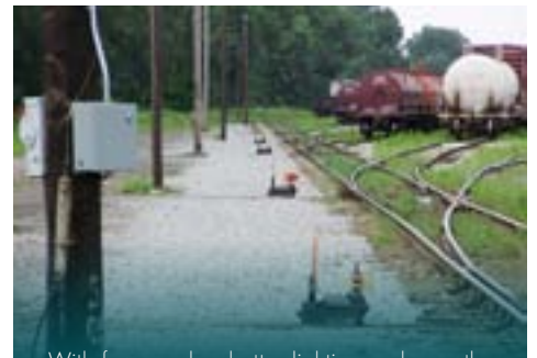
With fewer poles, better lighting and smoother walkways, Chicago South Shore crews enjoy an enhanced work environment at Burnham Yard.
